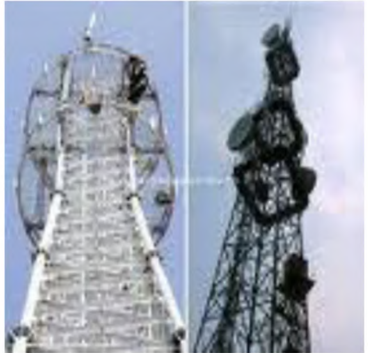
Fig. 6 Microwave tower for GSM Application
